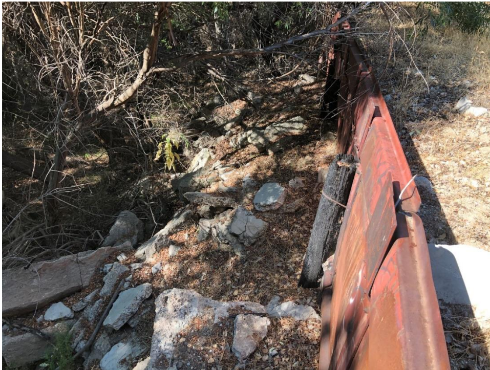
Photo 4. Typical construction waste debris supporting sheet metal flood wall with creosote pole tie-downs.
