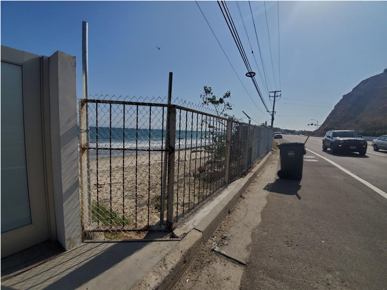
Photo 2: Unpermitted fence installed over existing fence – View of 21704 PCH
