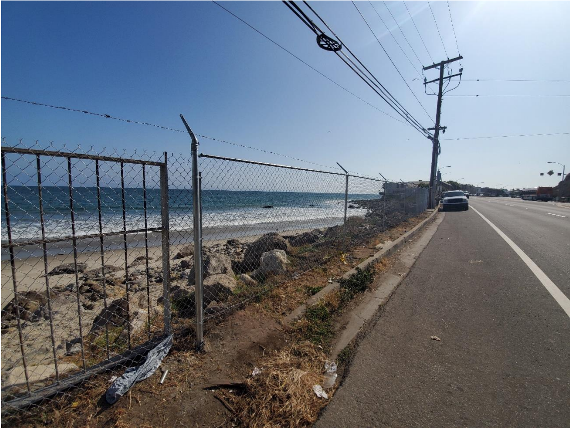
Photo 3: Unpermitted fence installed spanning both public parcels
